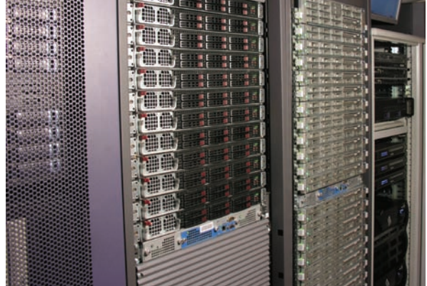
HPC hardware recently installed at MicroConsult
